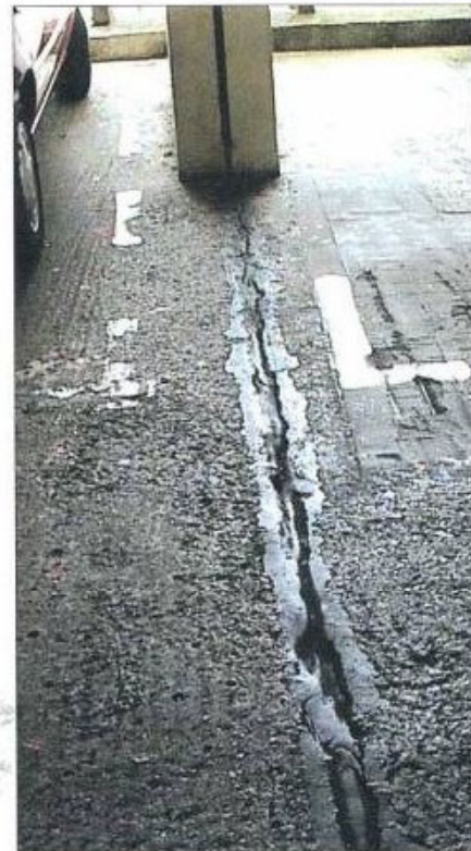
Ad hoc repairs are unlikely to slow the rate of deterioration
